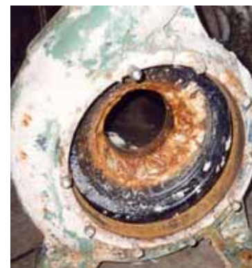
Repair old or corroded pump housing
